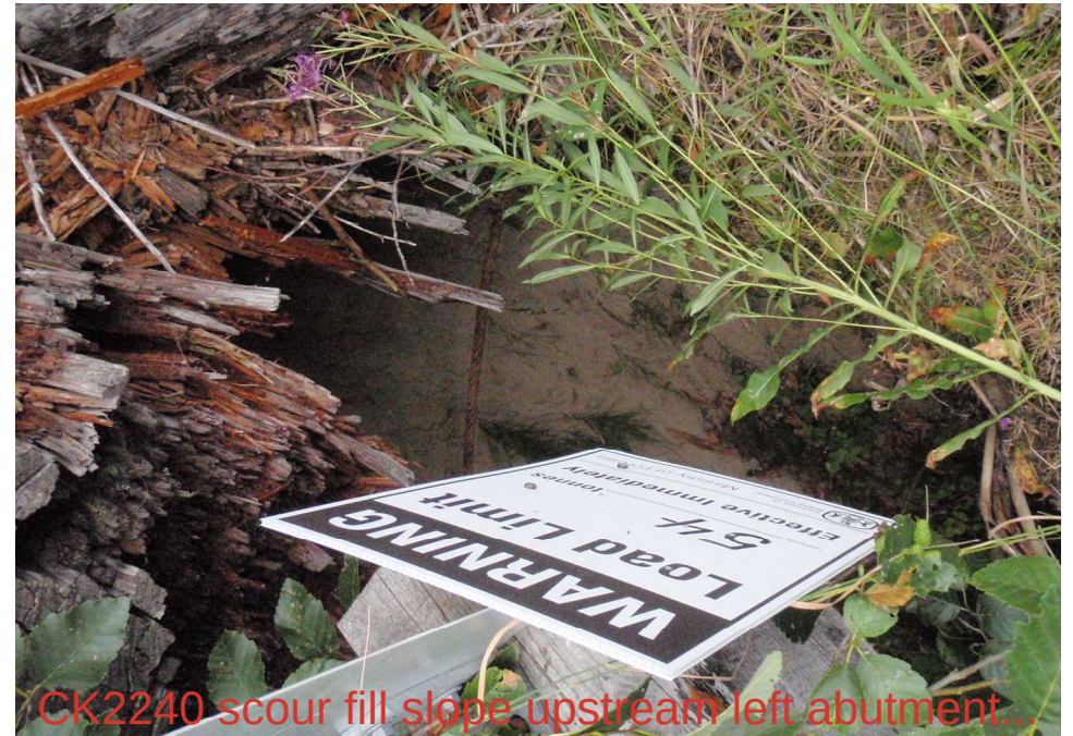
CK2240 scour fill slope upstream left abutment...
