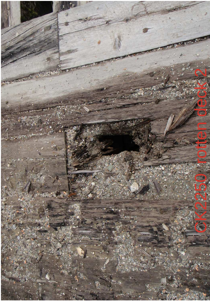
CK2250 rotten deck
