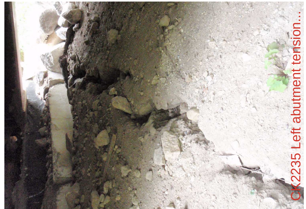
CK2235 Left abutment tension...
